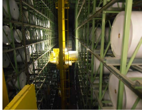
Figure 6, TransRoll roll storage is fully automated enclosed area without lights. Only the stacker crane's lifting platform has spot lights for the on-board video cameras
