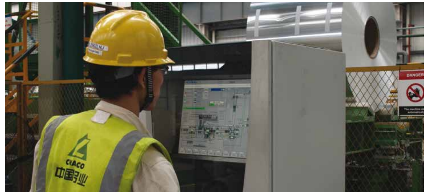
Line supervision is made with WinCC monitoring system
