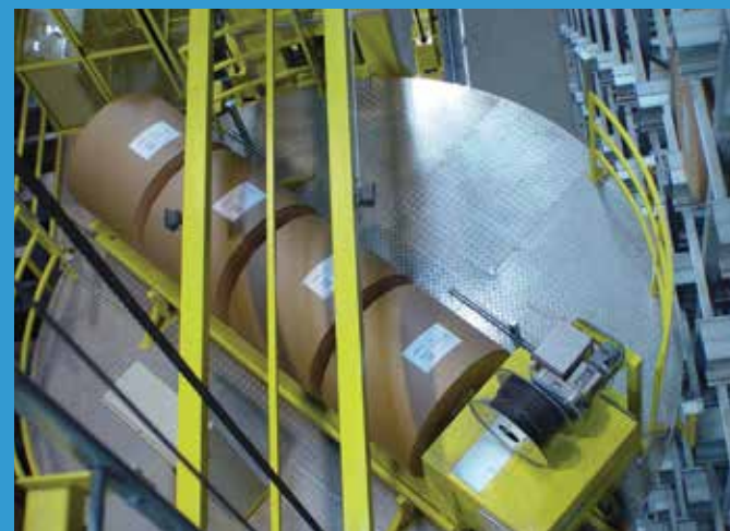
Load forming and sorting is done automatically by TransRoll® stacker crane.
